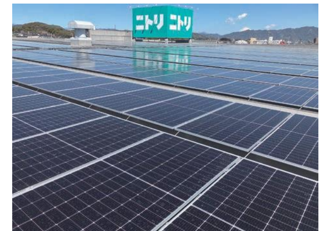
The solar panels on the rooftop of the Nitori Fujieda Store
