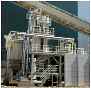
Pelletizing equipment turns collected particulate matter into pellets that can be reused as fuel
