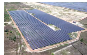
Power station exterior (drone aerial photo)
