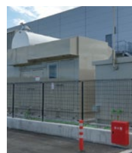
On-site power generation at Miyagi Distribution Center
