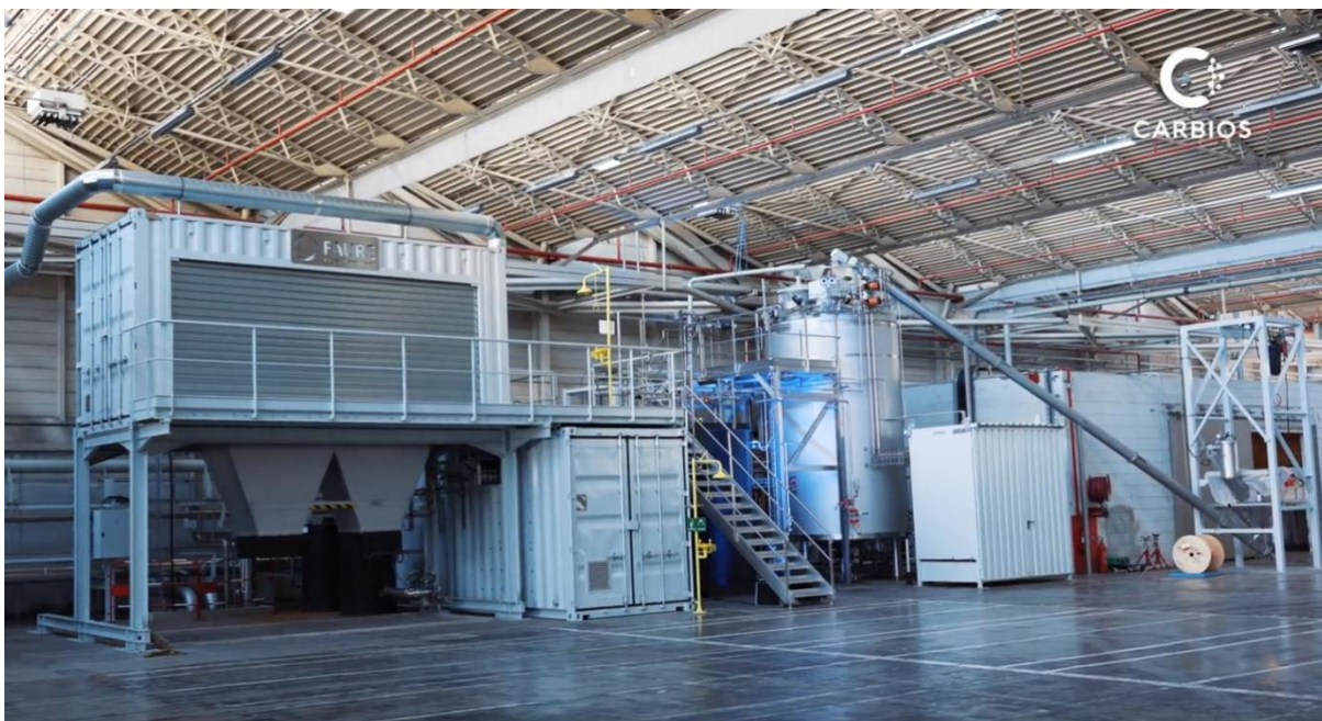
Partial view of the pre-industrial unit dedicated to the depolymerization of PET plastic and textile waste into monomers. (Carbios)
