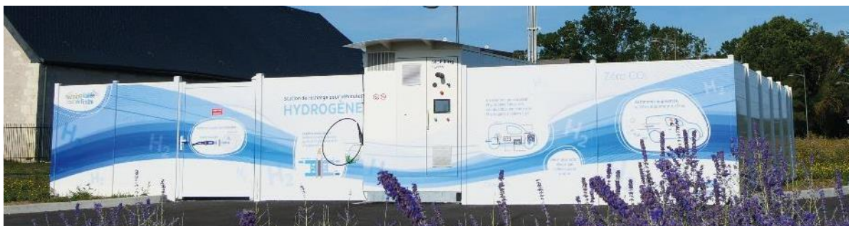
McFilling 20-350 hydrogen station in Sorigny
